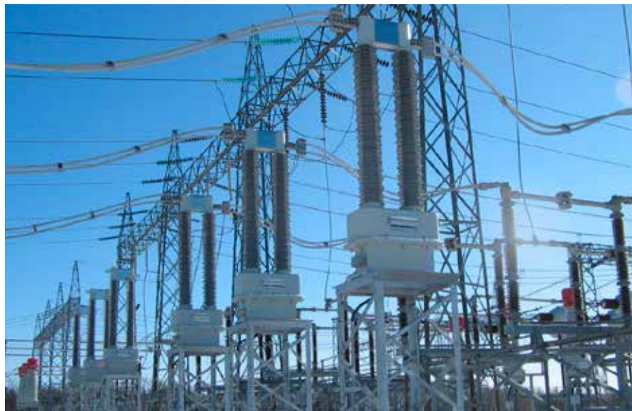
Figure 5 – 230 kV dry type current transformer installation in Central Canada
